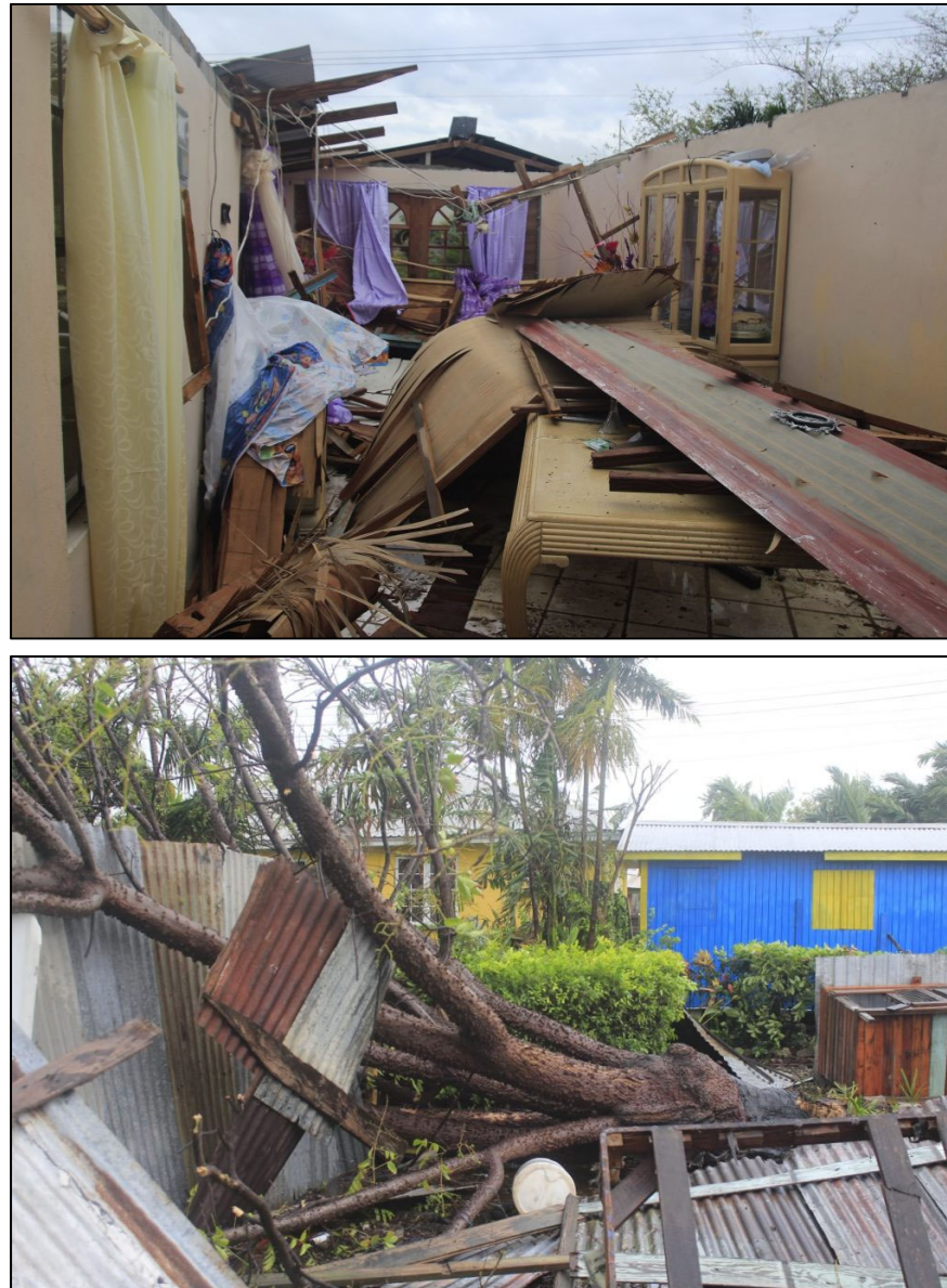
Figure 7. Example of damage caused by Elsa's hurricane-force winds in Barbados. Images courtesy of the Buzz-Caribbean news.
