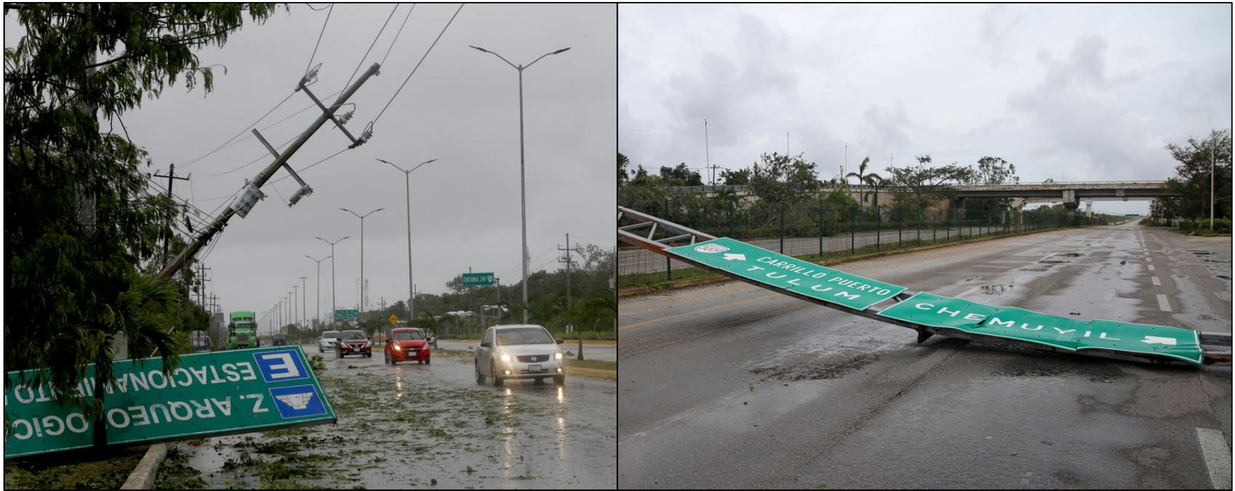
Figure 15. Hurricane Grace impacts in the Mexican state of Quintana Roo. Left: Damaged power lines and debris along a highway in Tulum. Photo credit: Marco Ugarte/ Associated Press . Right: A downed highway sign blocking a highway in Tulum. Photo credit: Paola Chiomante/ Reuters .
