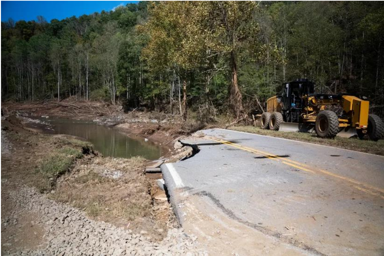
Figure 34. U.S. Route 19 in Yancey County is just one example of hundreds of roads that were washed out and destroyed in western North Carolina. Photo courtesy of Josh Morgan and USA Today.
