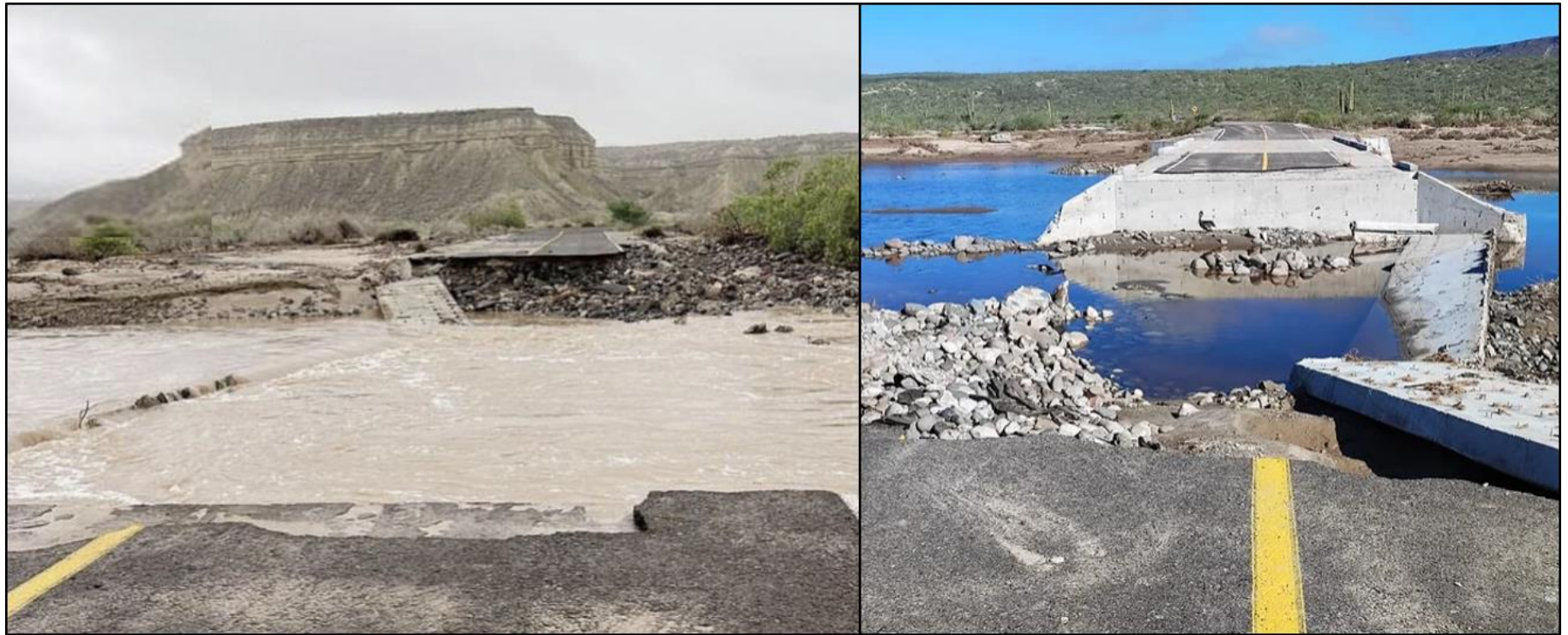
Figure 7. Roads damaged by flooding in the Comondú municipality of Baja California Sur. Image credits: (left) BCS Noticias and (right) Scorpion Bay Hotel, San Juanico.
