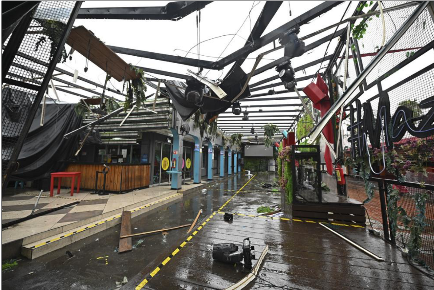
Figure 4. Wind damage in a commercial area in Mazatlán, Mexico. Courtesy of the Associated Press.
