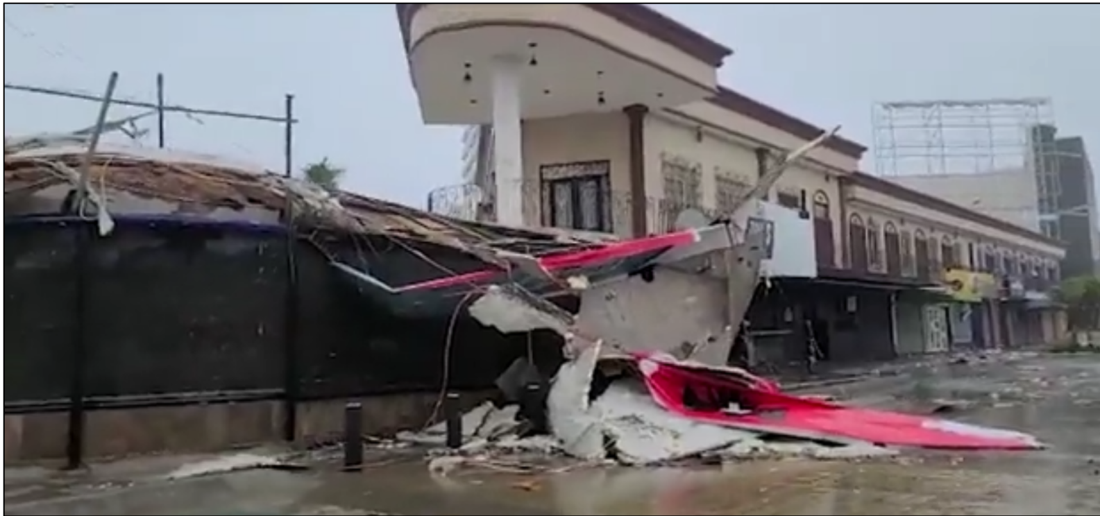
Figure 5. Image of damage to businesses in Mazatlán, Mexico. Courtesy of iCyclone.
